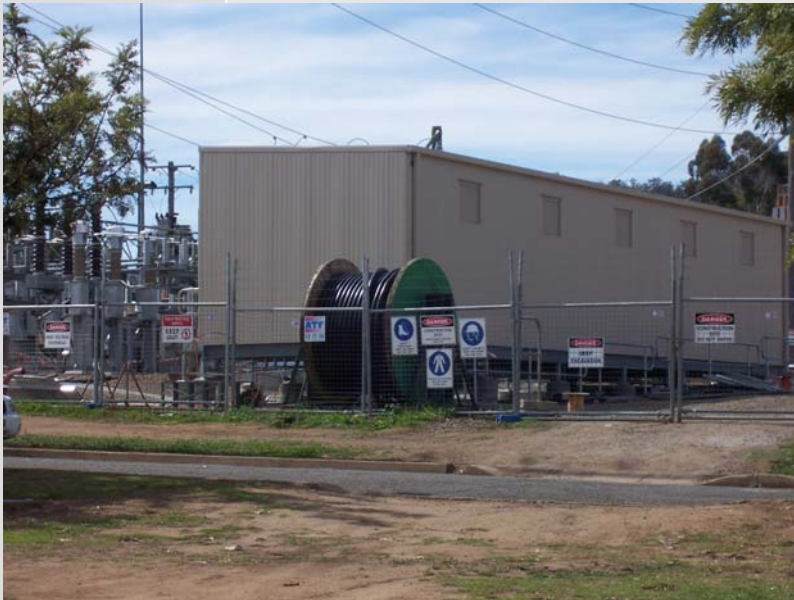
Above: The custom built transportable building after being transported to the East Tamworth substationsite
