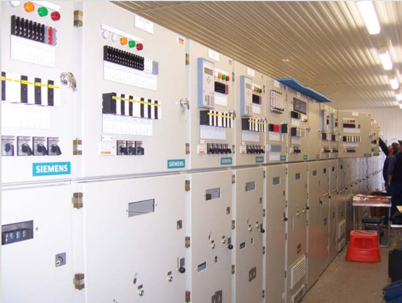
Above: The new Siemens Simoprime A2 switchboard after installation
